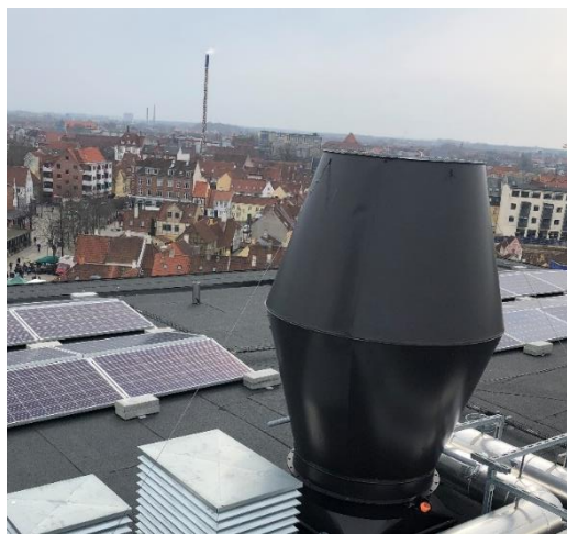
Air outlet from the kitchen
