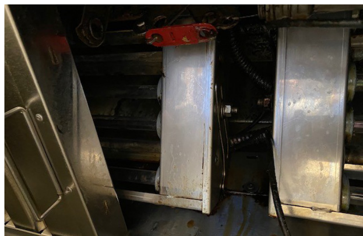
Grill - UV-C Lamps are placed behind the exhaust hood
